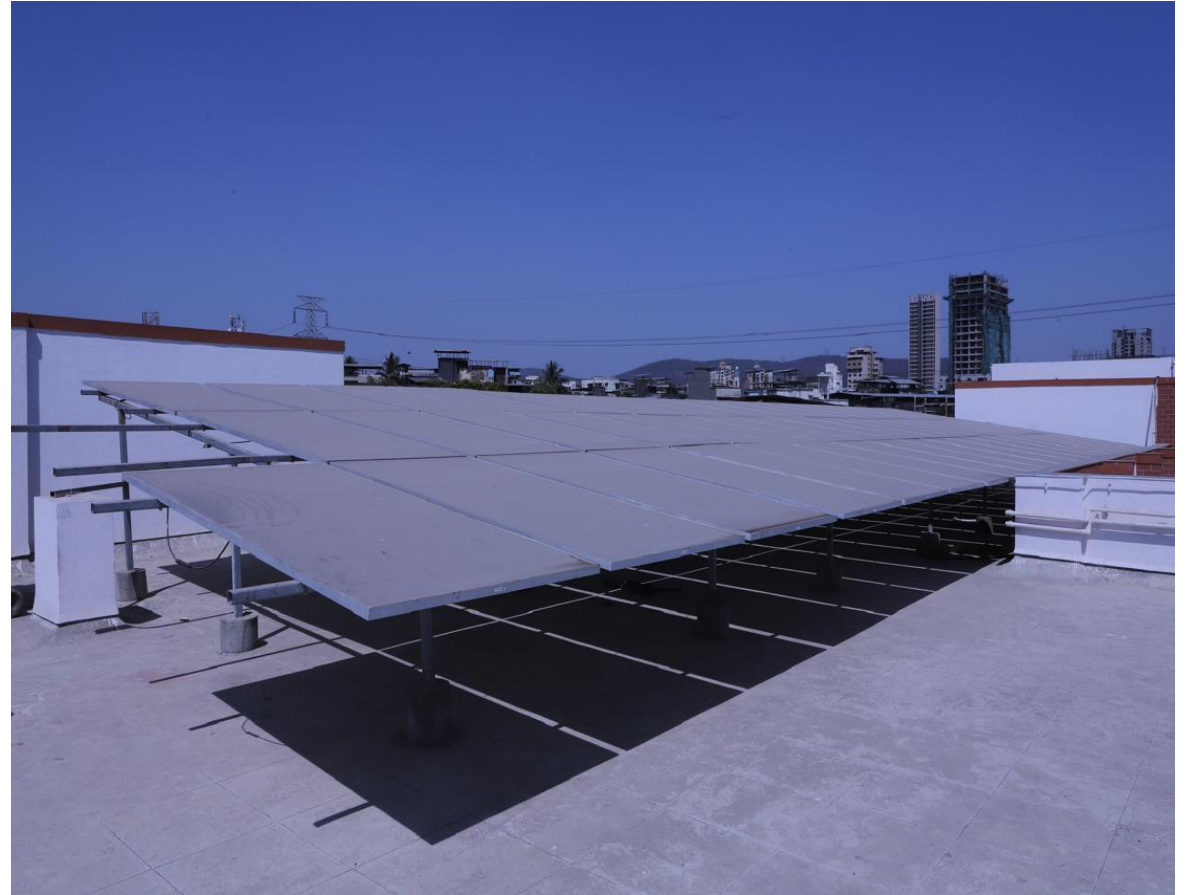
Solar Pannel On Terrace
